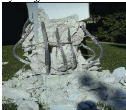
Figure 1: Failure at Construction Joint
